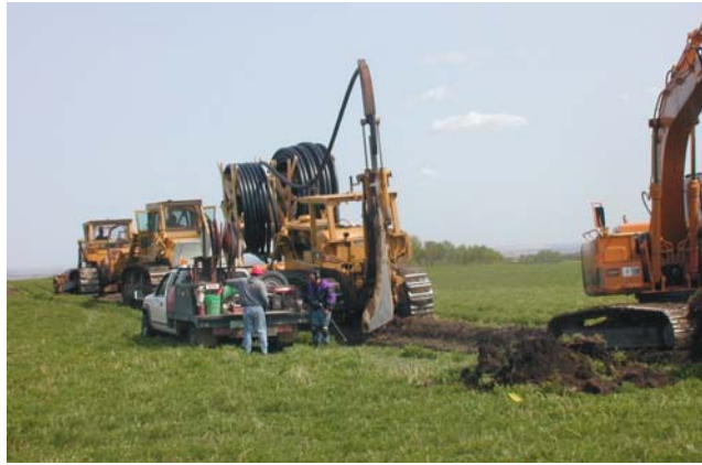
Figure 8. Trenching of rural water pipelines. Small diameter polyethylene pipeline trenching was adapted to prairie clay soils to supply farmsteads with water.
